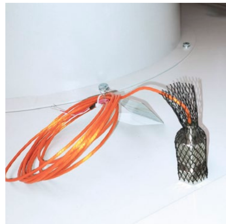
Fire Suppression System
